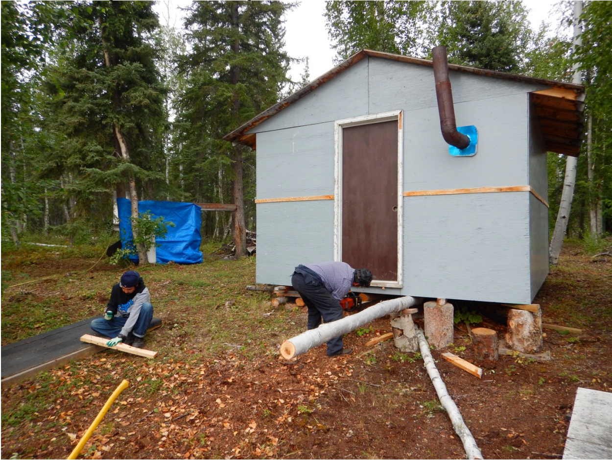
PHOTO 3. Lifting one of the cabins to get as close to level as possible. Photo By: Steve Olson
